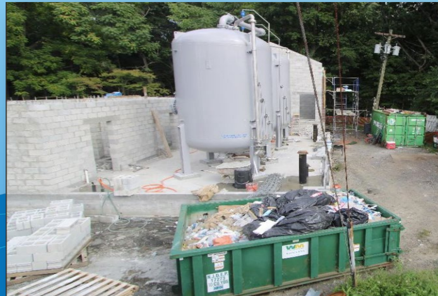
Ravine PFAS Treatment Facility
