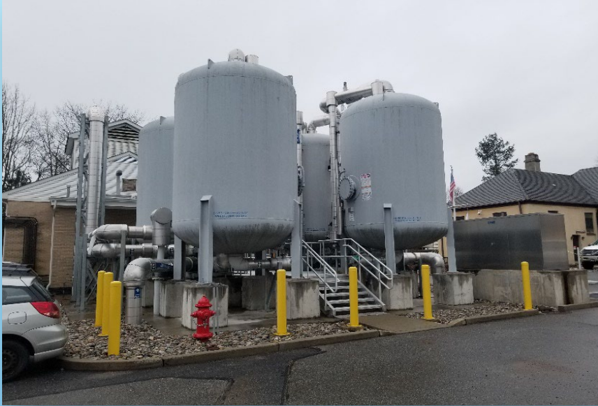
Carr PFAS Treatment Facility
