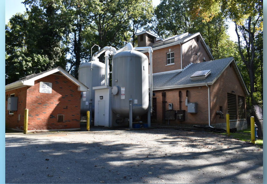
Twinney PFAS Treatment Facility
