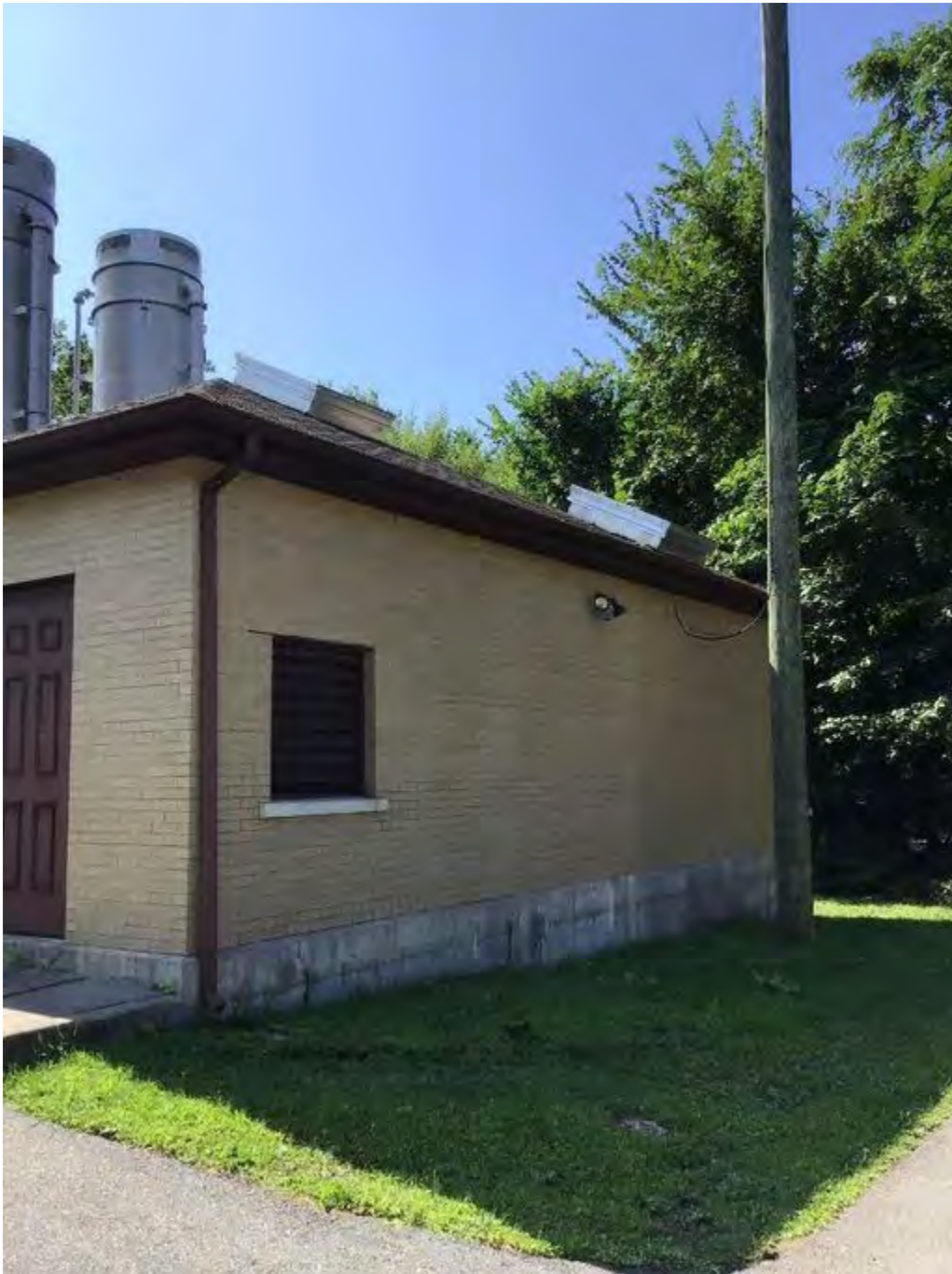
Roof hatches for pump replacement
